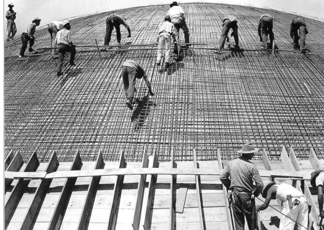
Construction of the building of the National Congress. Brasília, 1958. Acervo Fundação Oscar Niemeyer
