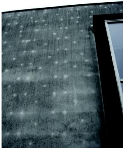
Figure 4 Typical pattern (in Europe often called “leopard pattern”) caused by the formation of fungi or algae on EIFS as a result of exterior condensation.
