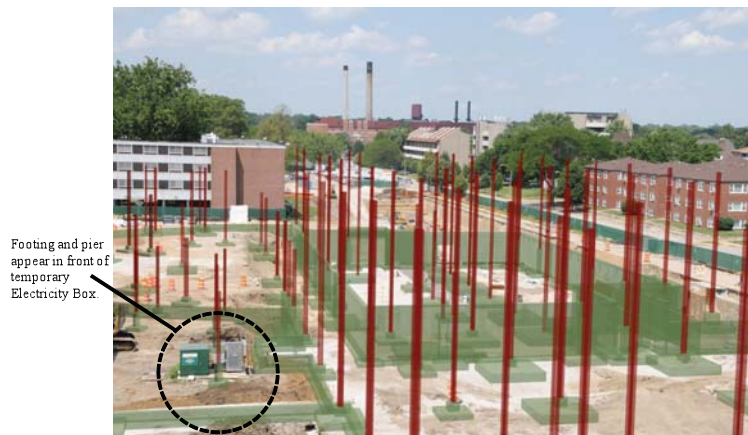
FIG. 20: As-built model superimposed over the progress photograph. Student Dining and Residence Hall construction project in Champaign, IL. Photograph courtesy of Turner Construction Company; Champaign, IL; used by permission.
