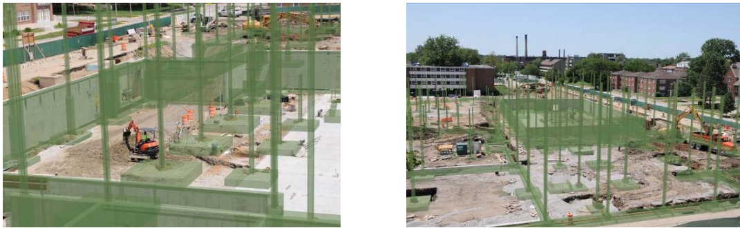
FIG. 14: The registration of images with the construction progress images. Student Dining and Residence Hall construction project in Champaign, IL. Photographs courtesy of Turner Construction Company; Champaign, IL; used by permission.
