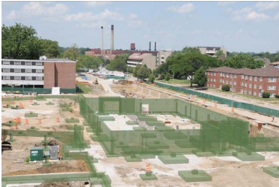
FIG. 12: The alignment of the Student Dining and Residence Hall construction project 3D model with one of the construction progress images using Golparvar-Fard et al. (2009) approach. As shown some of the foundations and foundation short walls as well as piers that are not yet constructed, are superimposed over the image. Photograph courtesy of Turner Construction Company; Champaign, IL; used by permission.
