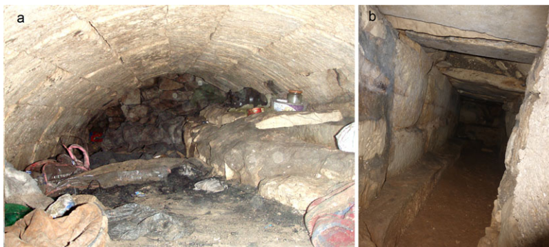
FIGURE 9 'Ein Qaryun tunnels. (a) Barrel-vaulted tunnel, 1.5 m wide; the shelf on the right is a secondary water channel. Note the blocking wall at the rear. Photo: Boaz Langford. (b) Tunnel built of large ashlar masonry at the left, stone slabs roof, with minor recent mortar repairs. Tunnel width is 60 cm. Photo: Ze'ev H. Erlich (Zabo) [Color figure can be viewed at wileyonlinelibrary.com ]
