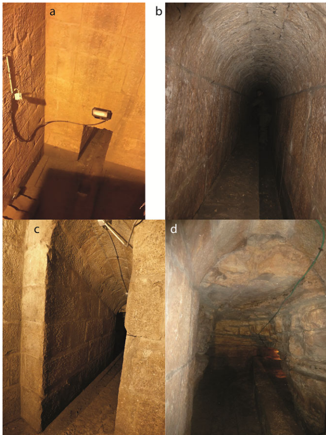
FIGURE 11 Ras el 'Ein water system. Photos: Ze'ev H. Erlich (Zabo). (a) The bottom of the entrance structure and the outlet toward Neapolis with high water level (wet year, spring 2015). Most ashlar courses are 60 cm high. (b) The barrel-vaulted built tunnel leading from the entrance structure toward Neapolis. Width of tunnel 75 cm. (c) The sloping vaulted roof tunnel connecting the bedrock tunnel and the entrance structure. Tunnel is 1.3 m wide. (d) Rock-cut tunnel draining the karstic spring system. Bedrock is well-bedded Eocene limestone. Tunnel is ca. 2 m wide [Color figure can be viewed at wileyonlinelibrary.com ]
