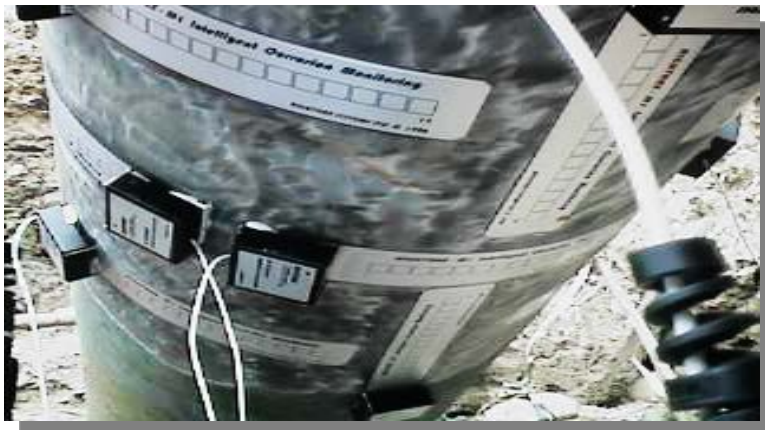
Multiple M1 Sensors fitted to subterranean Pipeline Prior to coating reinstatement and back filling
