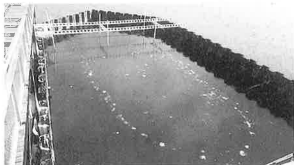
Excavation using a cofferdam: the wreck – visible as air bubbles – of the merchant brig designated YO 88 at Yorktown, Virginia, scuttled during the Revolutionary War.
