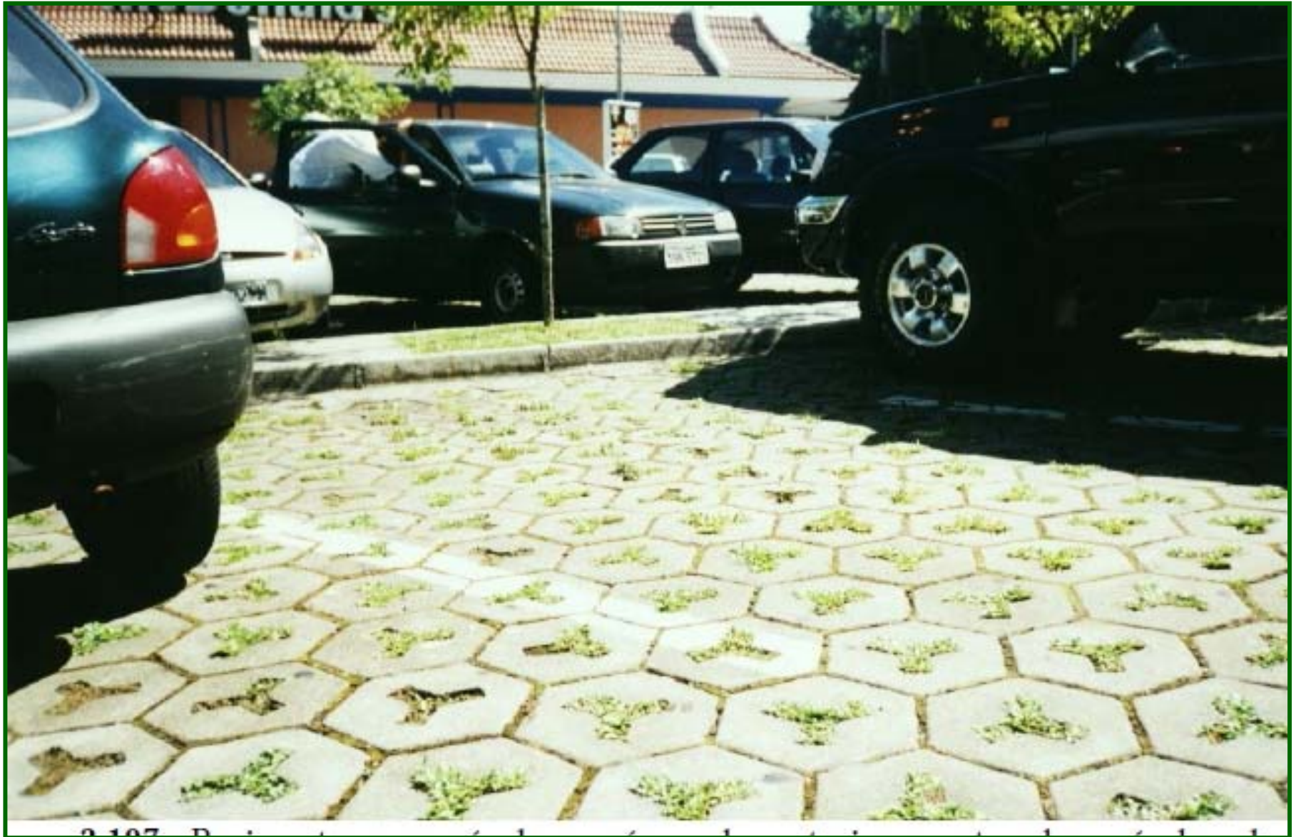
9-107. Paving stones with small plants growing in the gaps.
