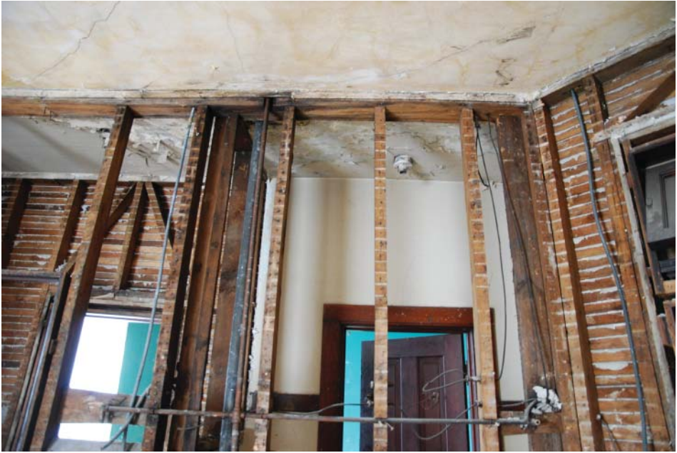
FIGURE 5 The ongoing renovation of the unoccupied upper floors of the Home allows archaeologists to study the changes made when the building was converted from a private home into a boarding house.
