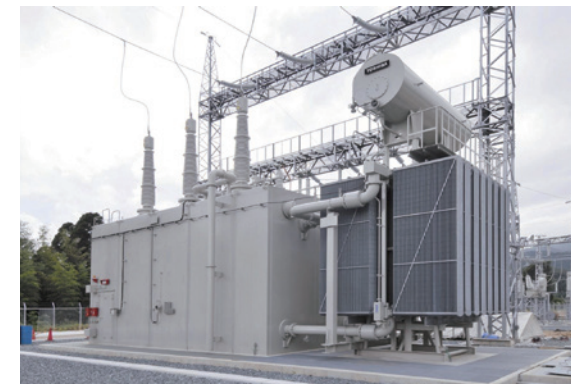
Roof-delta Connection Transformer
