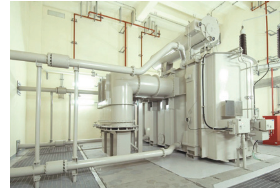
Scott Connection Transformer
