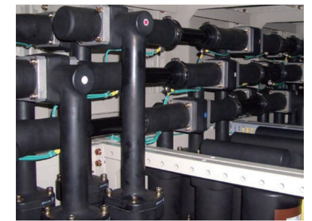
SIS Busbar Compartment
