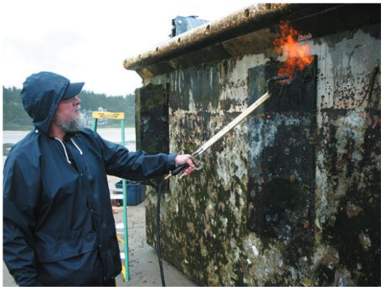
A worker in Newport, Oregon, burns debris off a Japanese concrete dock that washed across the Pacific.
