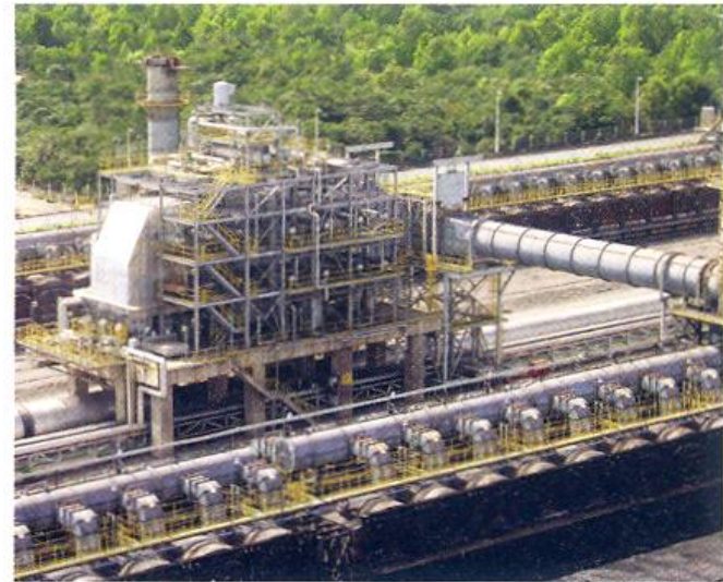
Figure 4. One of the heat-recovery boilers
